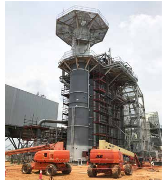
ERANOVE'S POWER PLANT PROVIDES ELECTRICITY TO THE EQUIVALENT OF 2 M PEOPLE IN TOGO
