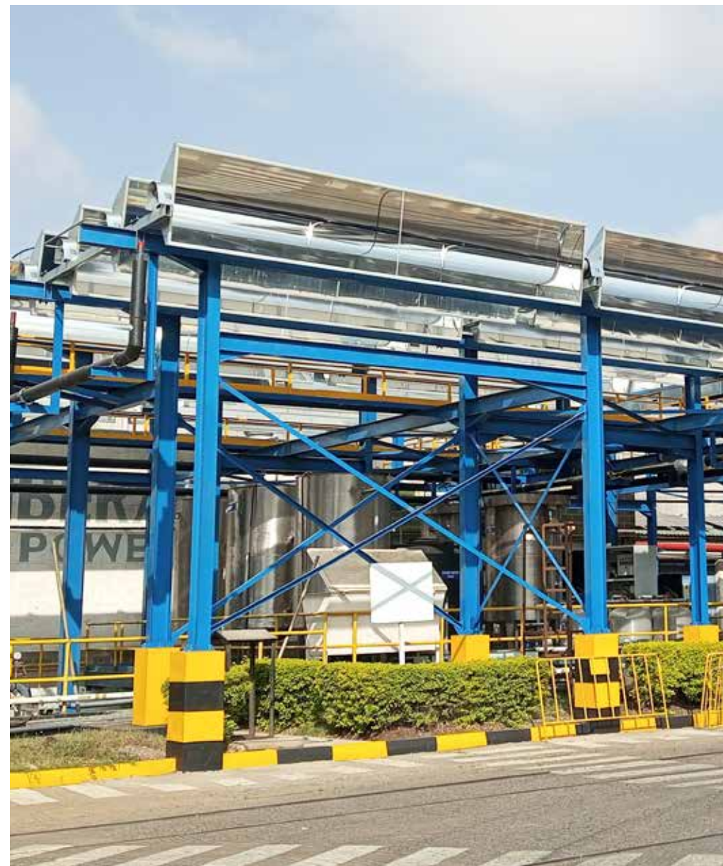
INNOVATIVE SOLAR HEATERS INSTALLED AT IBERAFRICA IN KENYA
